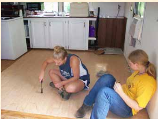
Lindsay works to install a new floor in a home on one of the worksites.
