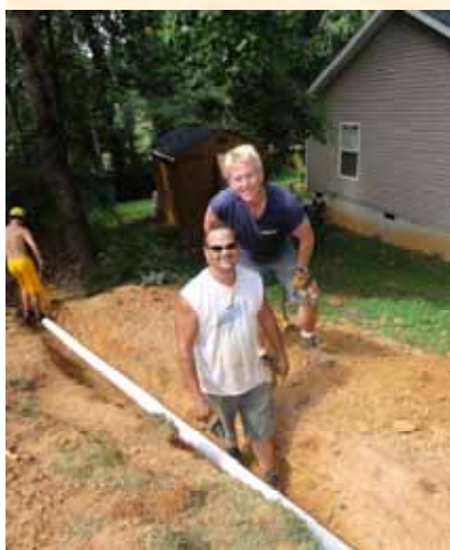
Dave takes a moment to pose for a picture while laying piping for a newly installed septic system.
